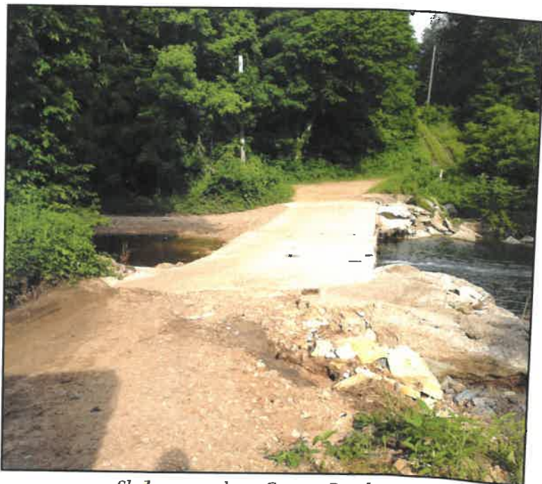
Slab approach on County Road 734
